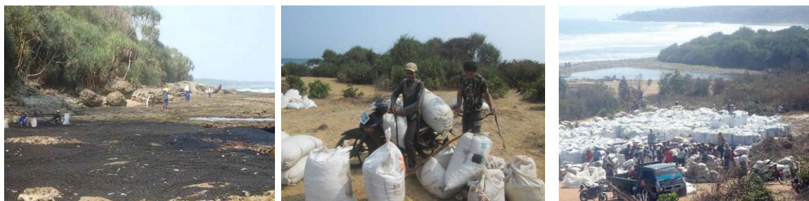
Left: Manually recovering the coal and storing it in bags; Centre: transferring bags to the primary storage site using small two-wheeled vehicles; Right: View of the primary storage site, a month and a half after the incident. The coal was to be evacuated in bulk bags by small trucks (Source: ITOPF)
