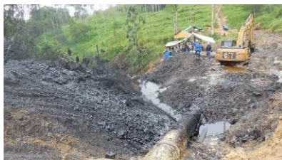
View of the leaking section of the Norperuano Pipeline (Source: OEFA)
