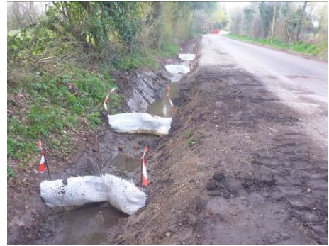
Series of custom-made devices (sorbent strands and wire mesh) to capture the residual pollution along a roadside ditch which the fuel had entered (ditch purged and scraped prior to installation of the devices) (Source: Cedre)
