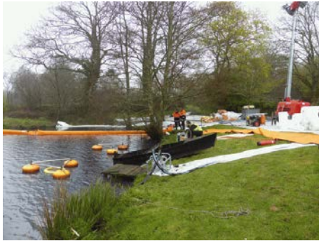
First pond: containment using floating booms and sorbent booms; recovery using mechanical weir skimmers. Note the ground protection with geotextile. (Source: Cedre)
